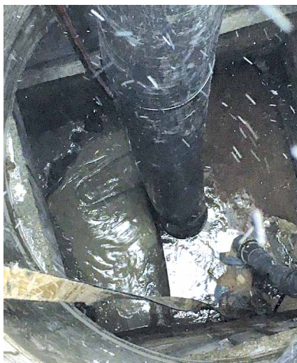
Figure 7. Frac-out in an Adjacent Manhole.
